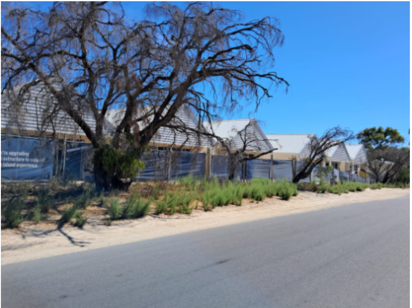
New staff housing underway at Rottneest Island (Photo courtesy of Ray Watson BWA Vice President)
